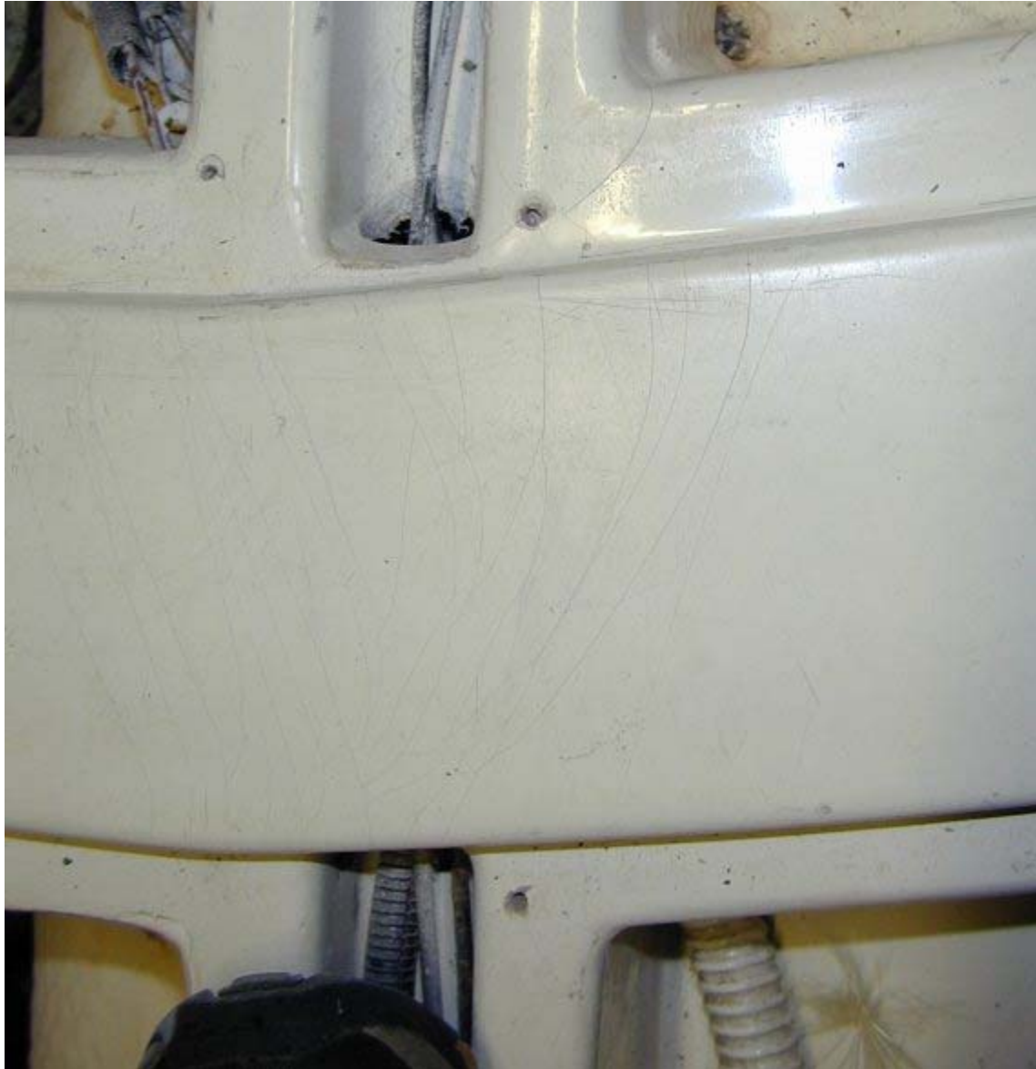
Stress cracks in keel floor caused by grounding.
