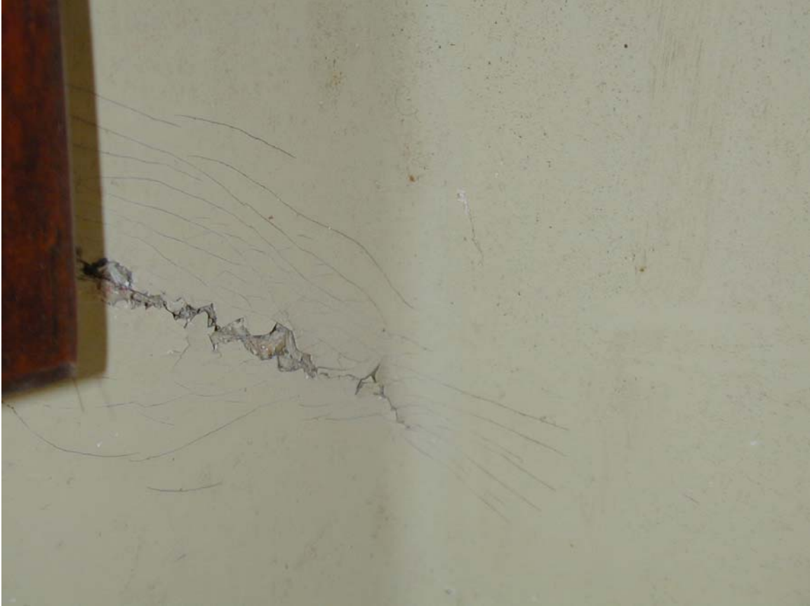
Fatigue cracks surrounding a crack through the laminate. Often found at the corner of a cutout.
