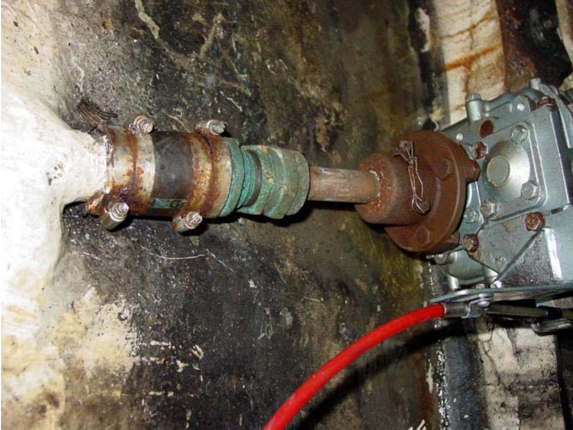
Typical stuffing box. This one needs a little love.
