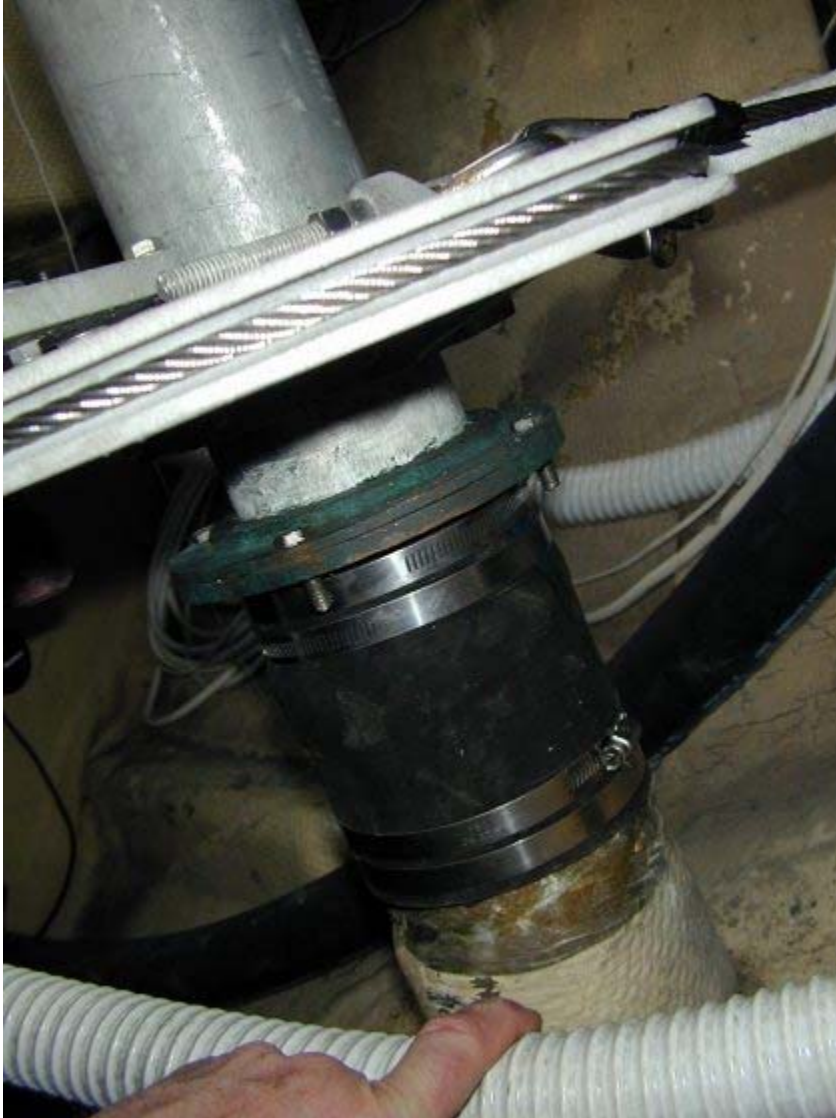
A typical rudder post stuffing box
